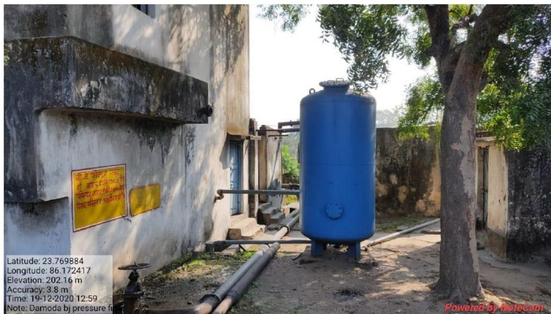
FILTER PLANT IN THE MINE AREA
